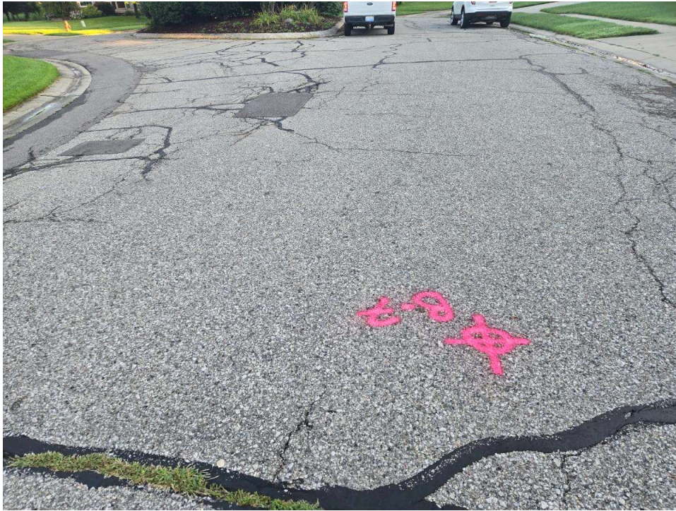
Photograph No. 7: Moderate to high severity transverse, fatigue, and secondary cracking with surface patching and crack sealing along Ancroft Court near boring B-07. View to the north.
