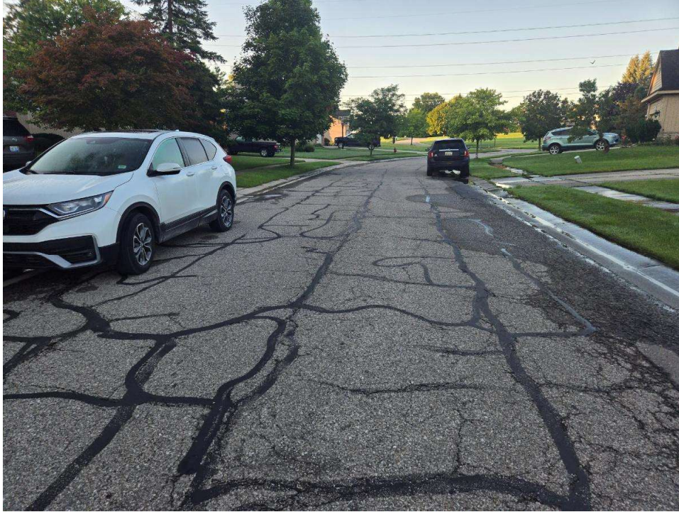
Photograph No. 5: Moderate to high severity transverse, longitudinal, secondary, and edge cracking with crack sealing along Berwick Drive near boring B-05. View to the south.
