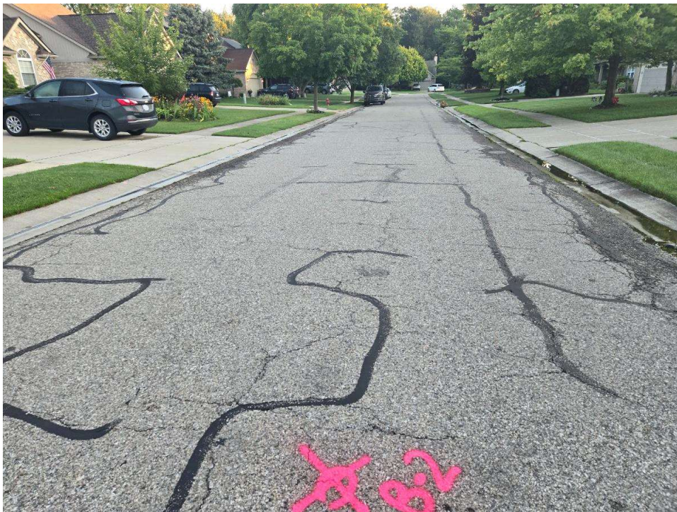
Photograph No. 2: Low to moderate severity longitudinal, transverse, and edge cracking with crack sealing along Adderstone Drive near boring B-02. View to the north.
