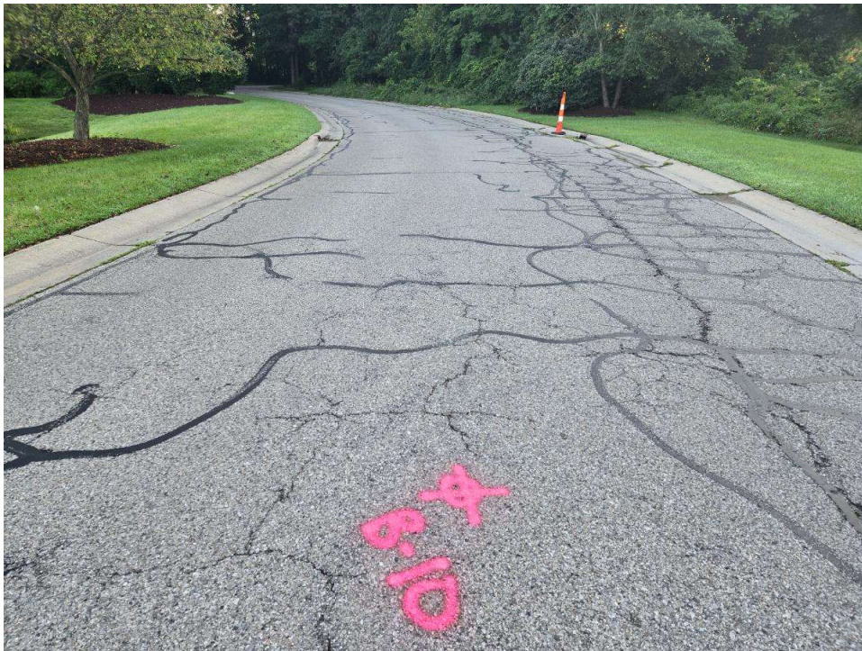
Photograph No. 10: Moderate to high severity longitudinal, transverse, and secondary cracking with crack sealing along Campfire Circle near boring B-10. View to the northeast.
