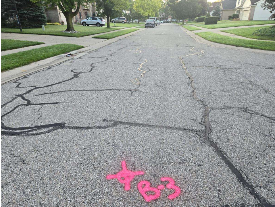
Photograph No. 3: Moderate severity longitudinal and fatigue cracking crack sealing along Berwick Drive near boring B-03. View to the east.
