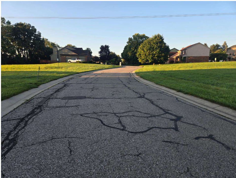
Photograph No. 6: Moderate severity transverse, longitudinal, secondary, and edge cracking with crack sealing along Golf View Drive near boring B-06. View to the south.
