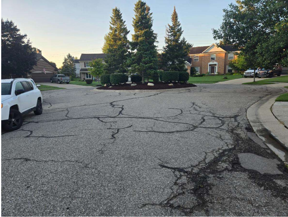
Photograph No. 9: Moderate severity longitudinal, transverse, and edge cracking with cold patching and crack sealing along Berwick Court near boring B-09. View to the south.
