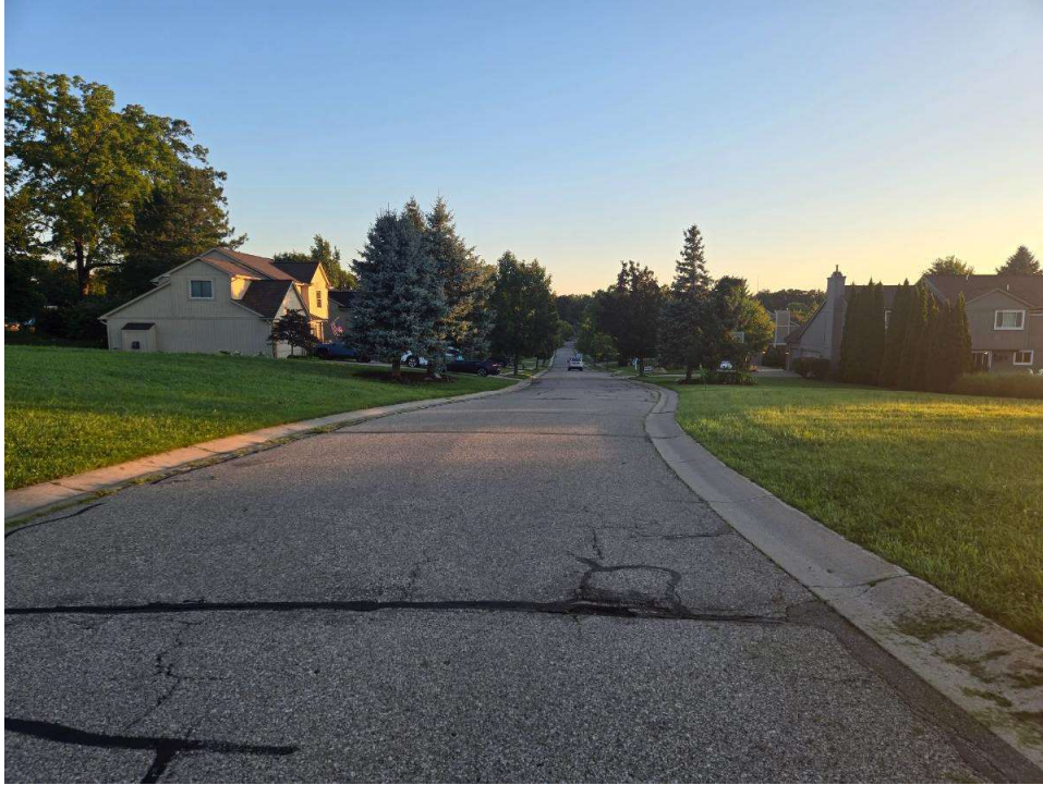
Photograph No. 1: Moderate severity transverse and secondary cracking with crack sealing along Adderstone Drive near boring B-01. View to the north.
