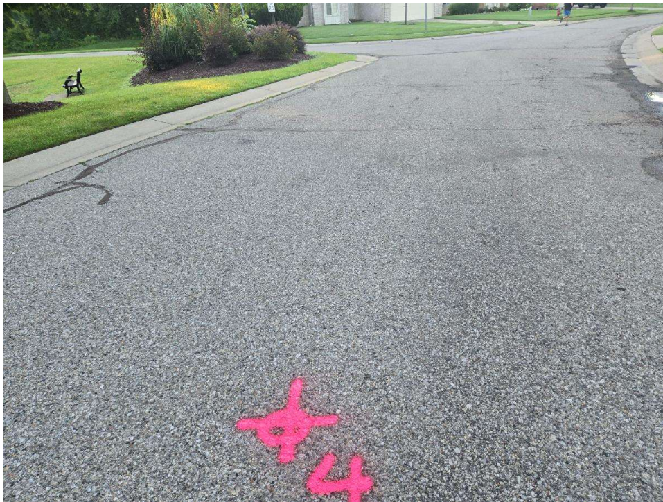
Photograph No. 4: Low severity edge and transverse cracking with crack sealing along Berwick Drive near boring B-04. View to the southeast.
