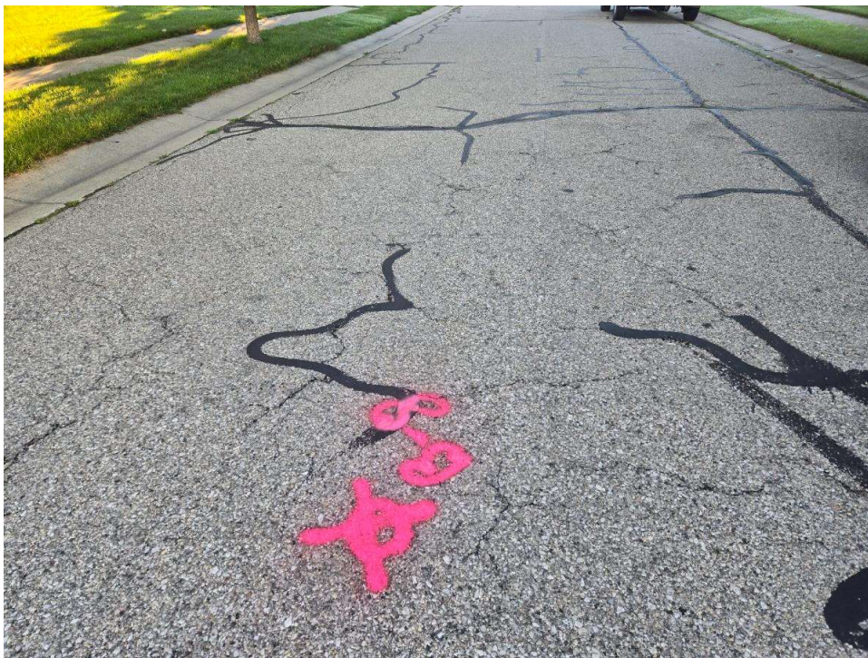
Photograph No. 8: Low to moderate severity transverse, longitudinal, and secondary cracking with crack sealing along Ancroft Drive near boring B-08. View to the west.
